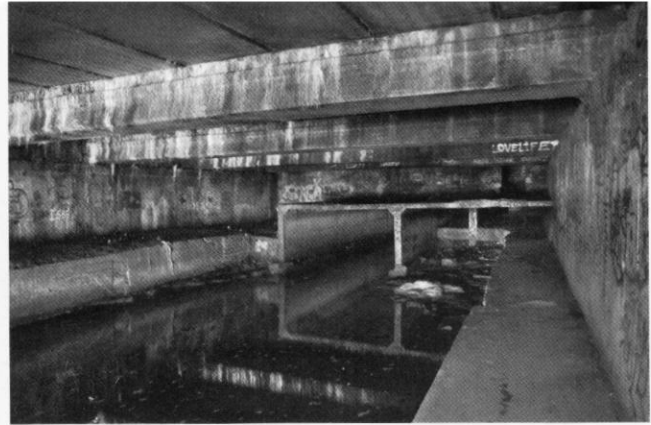
Entrance showing raised floor of air raid shelter section of the Ouseburn culvert
